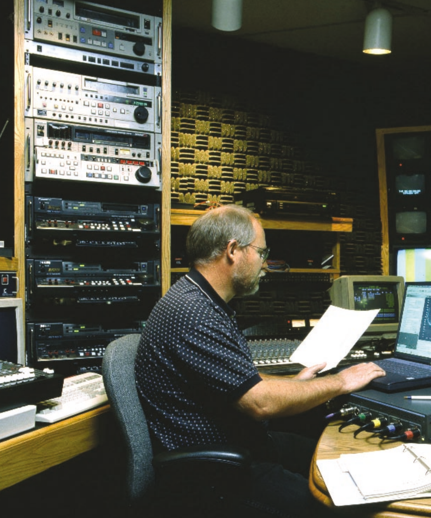
Pat Shearer, chief engineer at KWBP in Beaverton, OR, monitors the quality of the station's audio signals from the studio control room.
